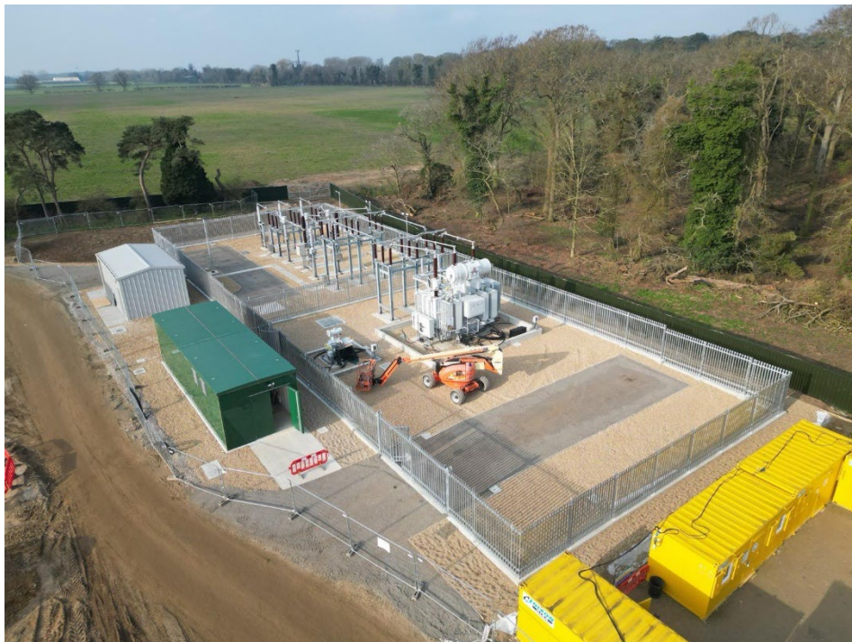
Image 5 132/33kV Substation (single transformer)
