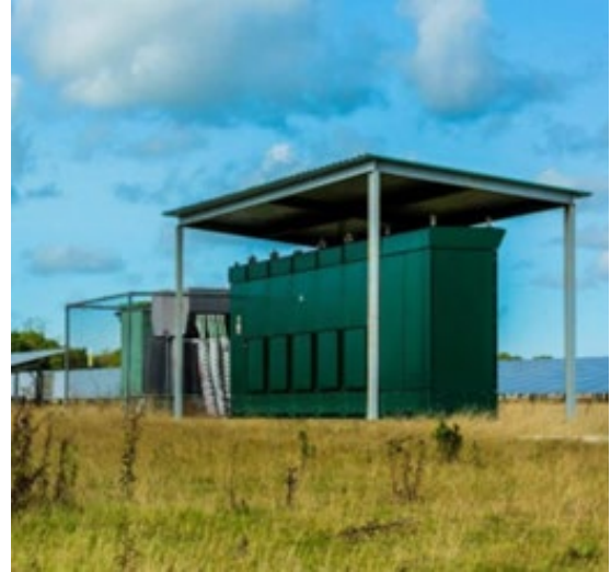
Image 4 Central Inverter Unit
