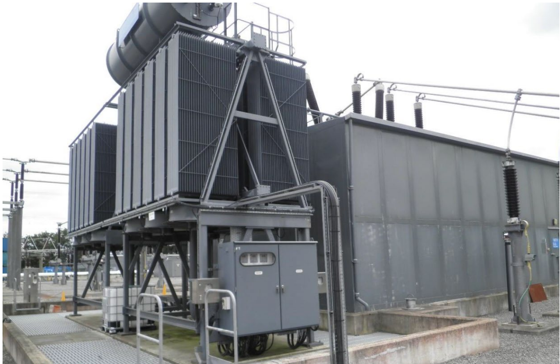
Image 6 Typical 400kV power transformer
